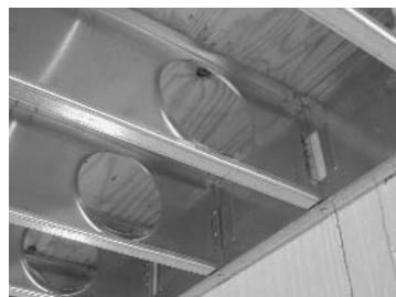
SIMPSON HANGER STEEL FLOOR
